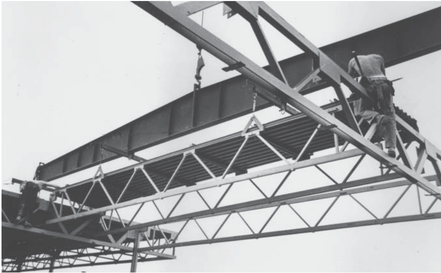
Figure 1.17 Steel deck is designed as the top chord of prefabricated open web steel joists. Courtesy of Inland-Ryerson Construction Products Company.
